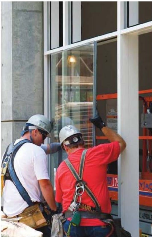
At the High Museum of Art (Atlanta, Georgia), this insulating glass unit (IGU) will rest on resilient, permanent shims called setting blocks and be centered in its frame by edge blocks. Temporary shims may be used to hold the unit tight against the interior gasket while the exterior gasket is applied.
